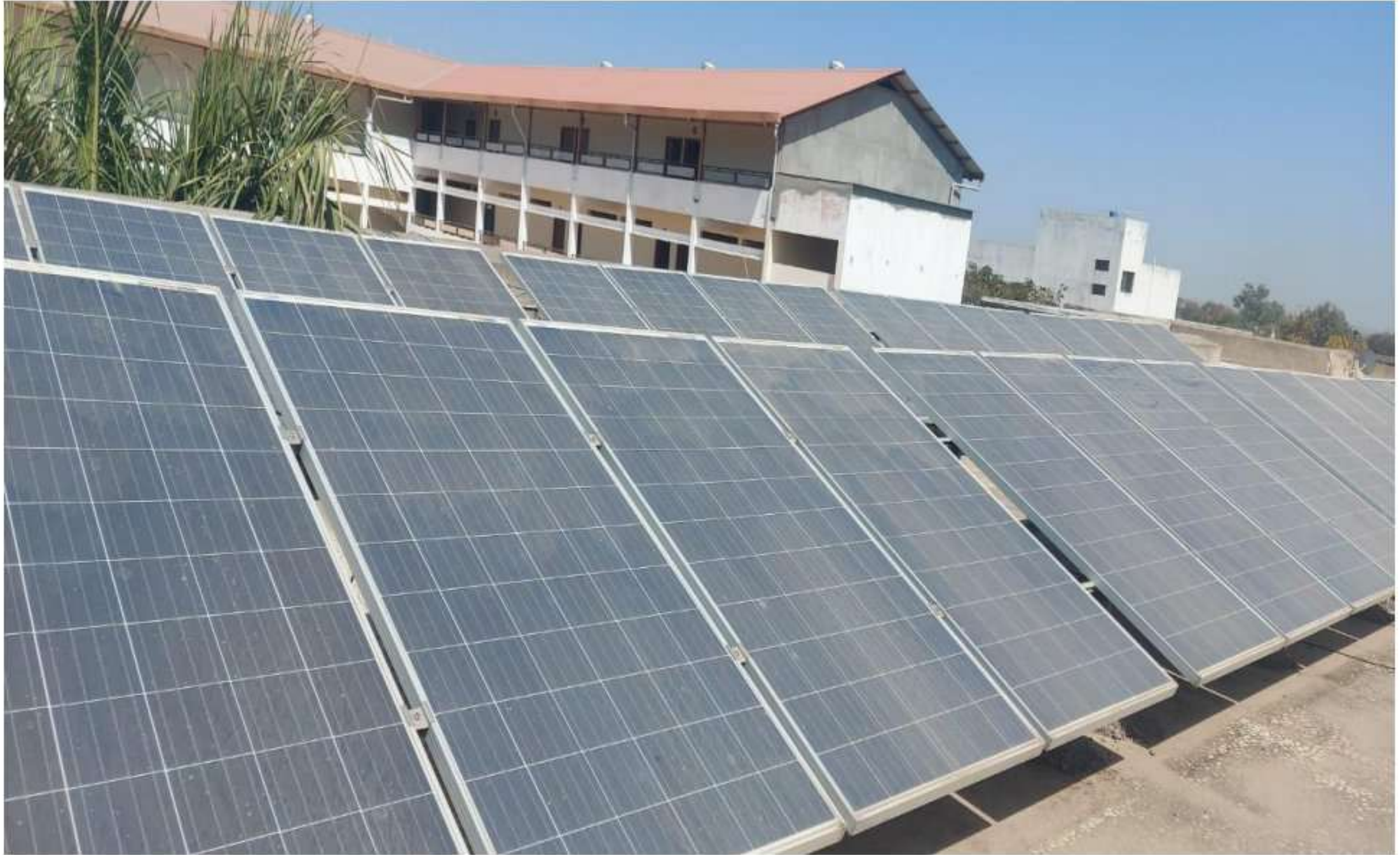
SOLAR POWER PLANT
