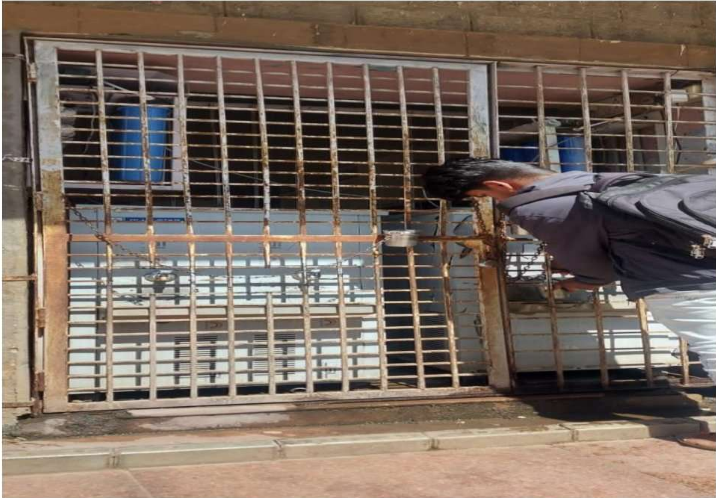
RO PLANT FOR DRINKING WATER
